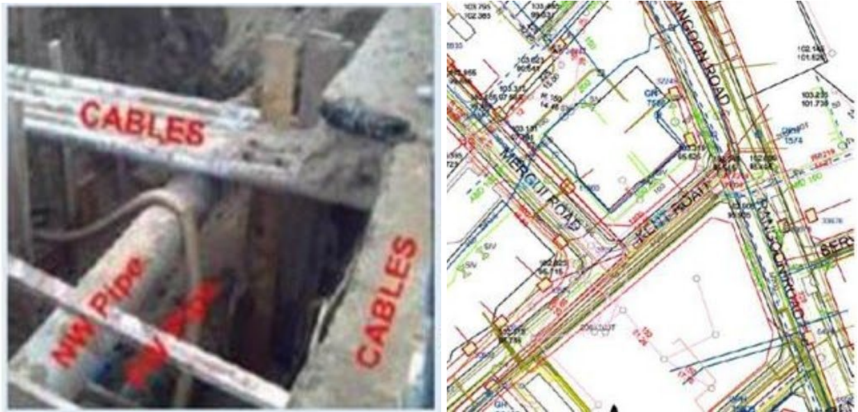
Messy arrangement of utility cables
